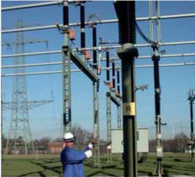
ASP non-contact voltage detector used in an outdoor switching station.
