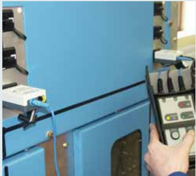
Use of DEHNcap/PC-LRM phase comparator with two HR-LRM test adapters for an HR switchgear installation.
