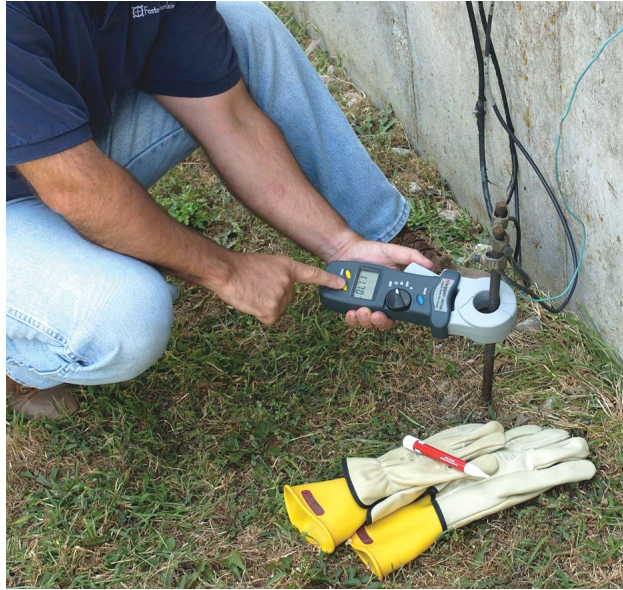
The DET20C instrument is shown being used to test a facility ground.
