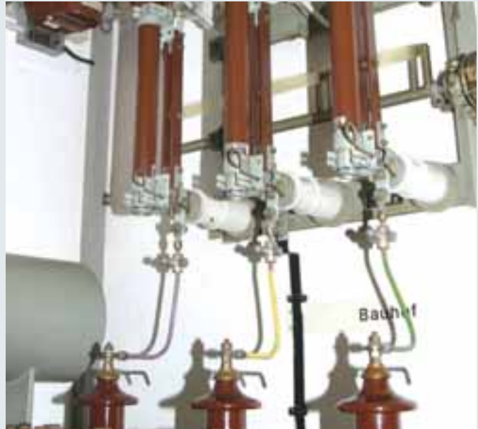
Fixed ball point attached to the round copper conductor of a switchgear installation.
