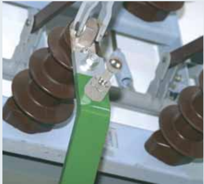
Straight fixed ball point installed on a busbar.
