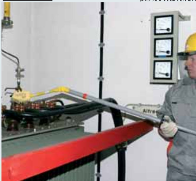
Damp cleaning of a transformer using the FRS ZK MS damp cleaning kit.
