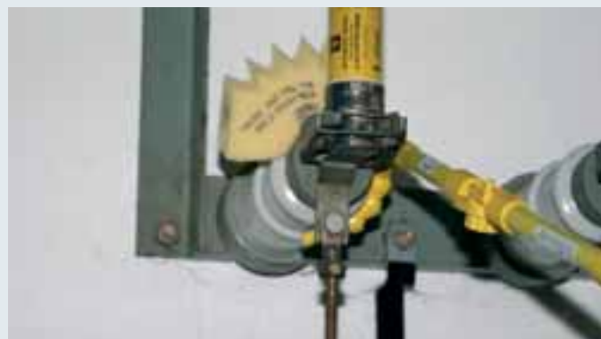
Damp cleaning of an insulator with a dual operating head.
