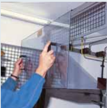
Inserting an insulating protective shutter (transparent), type A2.
