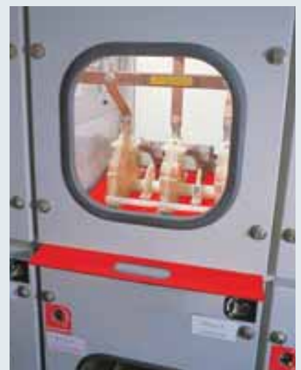
Inserting an insulating protective shutter, type A4.
