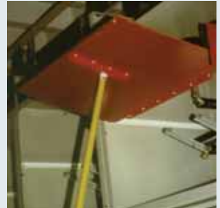
Inserting an insulating protective shutter, type A3, by operating rod
