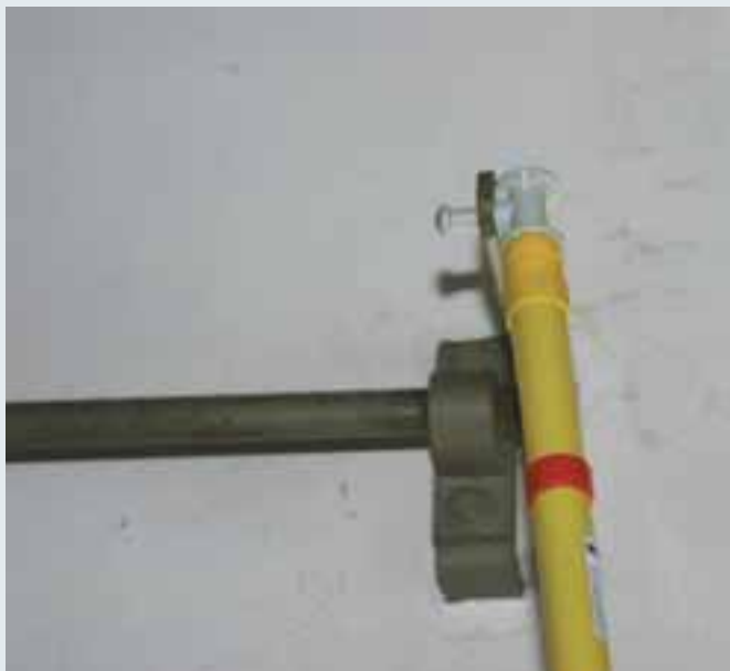
Switching a disconnector by means of an IS SK insulating rod with switching rod head.
