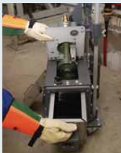
After lifting the conveying pump out of the HT mass, the oil reservoir can be removed for refilling.
