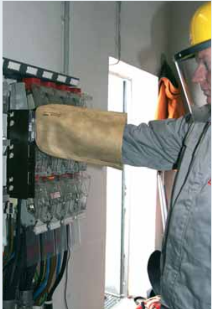
Inserting an NH fuse using the required personal protective equipment.
