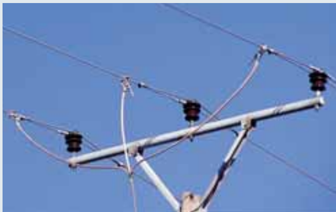
Phase screw clamps used on an overhead line.
