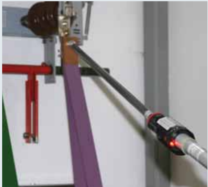
PHE III voltage detector with visual and acoustic indicator used on an indoor switchgear installation.
