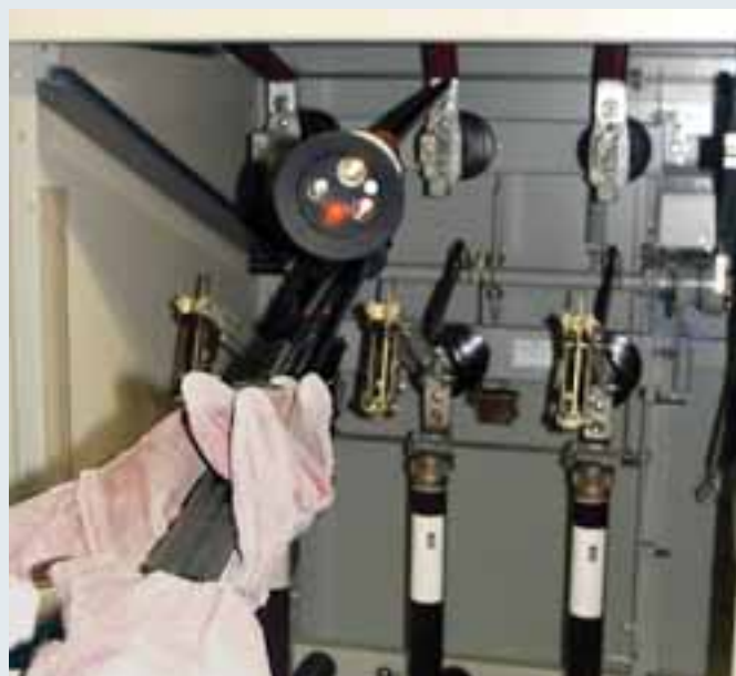
Single-pole PHV I phase comparator used at a switchgear installation.
